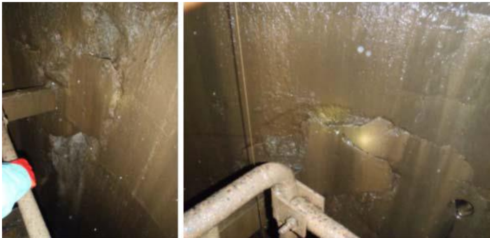
Fig. 2 Damaged places on the blind shaft
